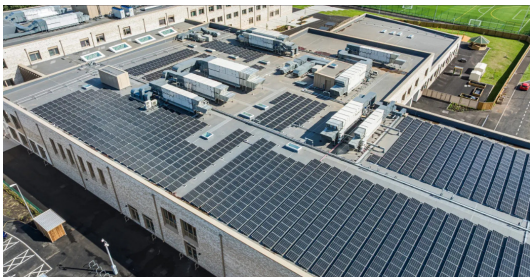
Fig. 6. Rooftop photovoltaic array, Drumgeith Community Campus/Greenfield Academy (source: Goodson Associates)
