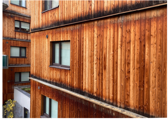
Fig. 11. Aspern D12, Black mold on a fire-protection profile in a facade system, 2024
