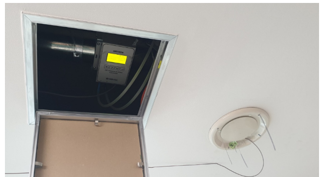
(b) Supply diffuser and flow metering equipment
