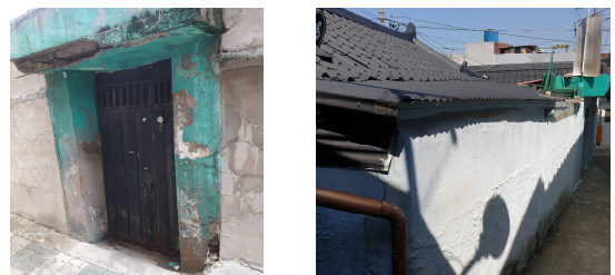
Fig. 2. Deterioration of the physical environment at the research site
