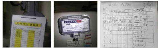
(a) Energy monitoring device
