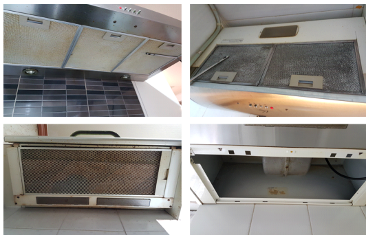
Fig. 3 Maintenance problem for Range hood
