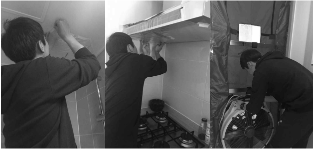
a) Sealing the ventilation b) Sealing the hood c) Install the blower door Fig. 4. Sealing leakages and installing the device
