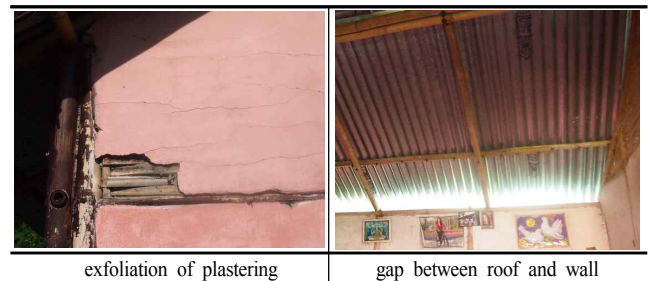
Fig. 5. Problems of houses provided by Habitat for Humanity, Nepal
