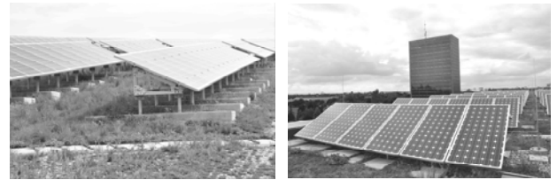
Fig. 17. Examples of PV installation on green roof in foreign
